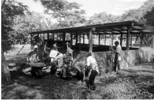
Escalante community members work on grading outside the new school. Construction costs were funded with a $2000 donation from a SCP supporter.
