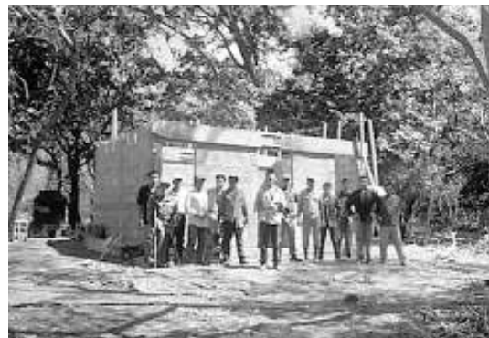
The Health Center in La Palma was built with volunteer labor by Association members.
